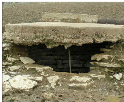
Figure 3. This abandoned well is located in an agricultural area that is void of vegetation that could filter pollutants from stormwater runoff and reduce the amount of pollution entering groundwater resources.
