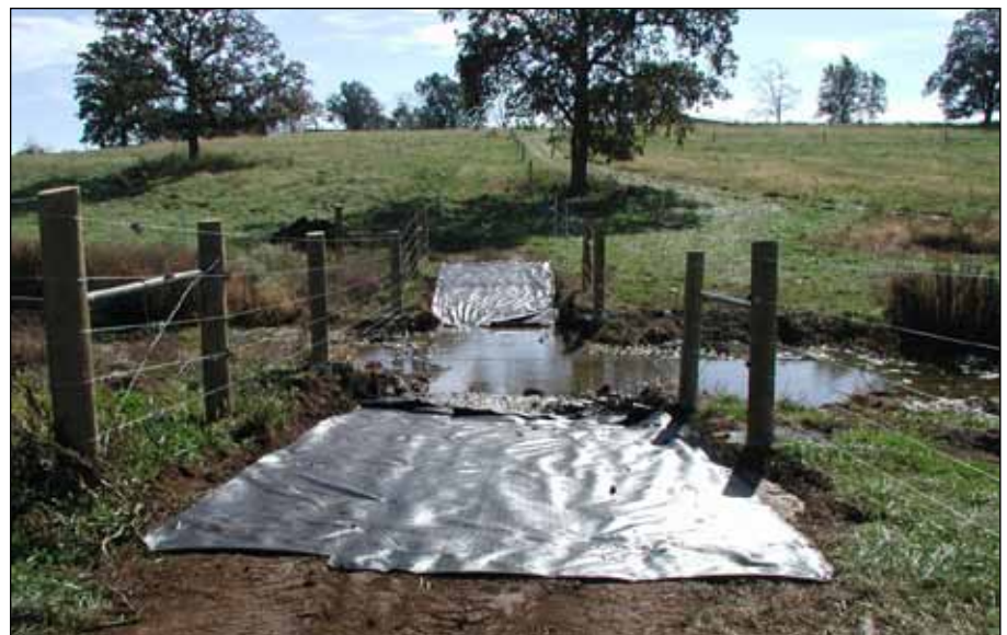
Figure 3. Once geotextile fabric is placed, it should be pulled tight, smoothed, and secured.
