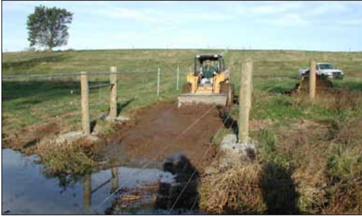
Figure 2. Use of a skid loader to grade the entrance and exit approaches of a stream crossing for a small stream. Grading provides a base for the geotextile fabric. Note the absence of rocks and debris on the approaches.
