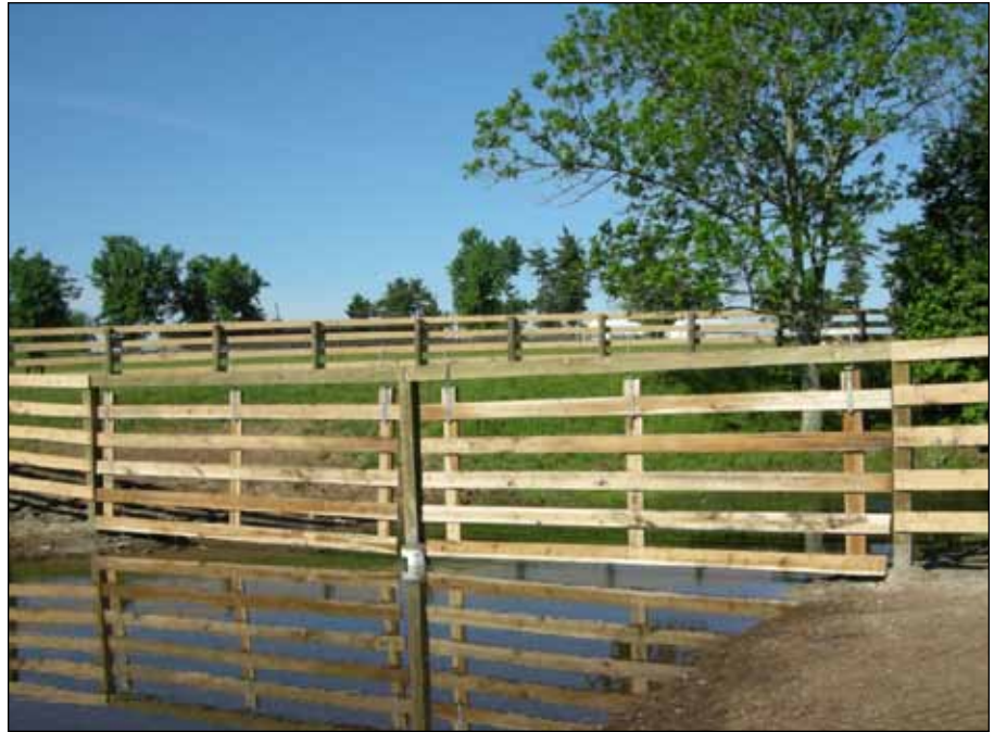
Figure 8. Swinging floodgates allow debris passage during high flows.
