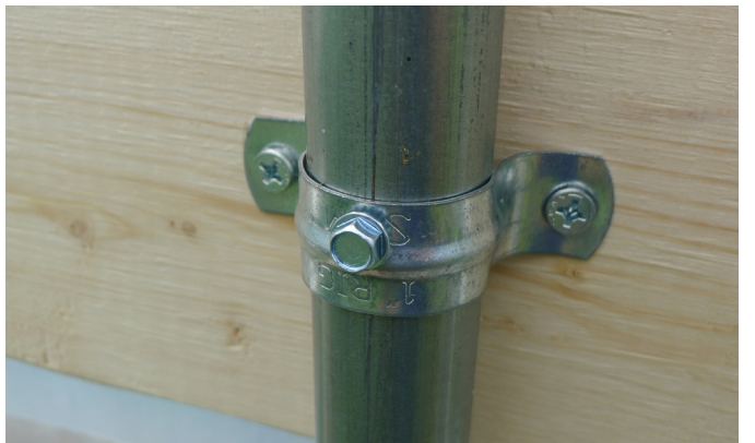
Figure 9b. Bracket and self-tapping screw attach gutter support board to tunnel bows.
