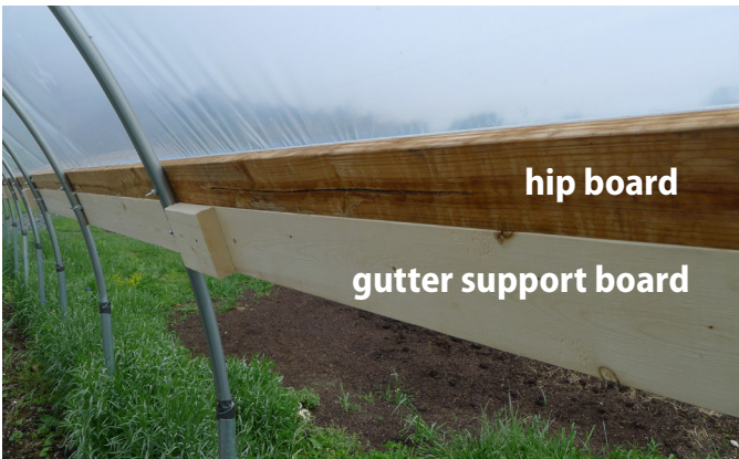
Figure 9a. Inside view of hip board and gutter support board.
