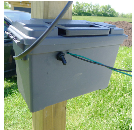
Figure 27. Plastic "ammo" box used to house battery, solar controller, fuse, switch, and electrical connections.
