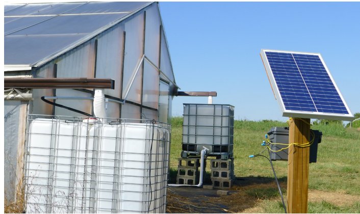
Figure 30. Rainwater collection and ultra-low pressure drip system on a tunnel at the UK Horticulture Research Farm. Solar pump is used to transfer water from the low tank (foreground) to the higher one.
