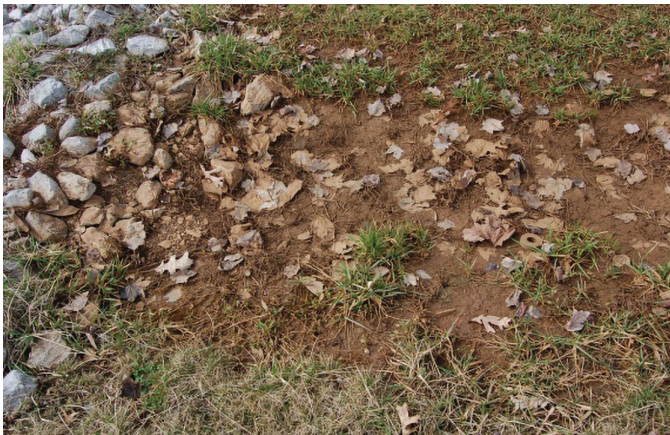
Evidence of sediment deposition next to riprap. Excess sediment reduces stormwater infiltration into the underdrain.
