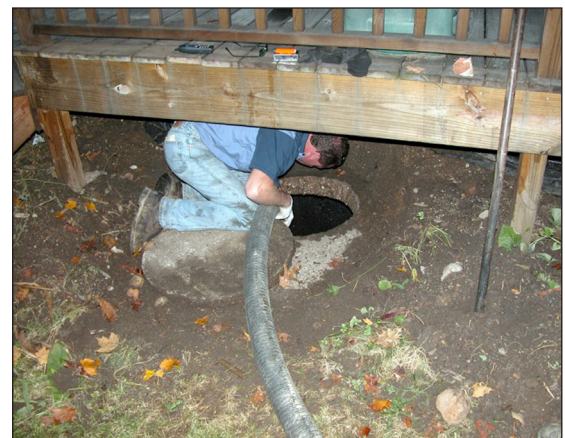
Figure 4. Septic tank located under deck being cleaned by professional. (Photo by Jeff Volenec)
