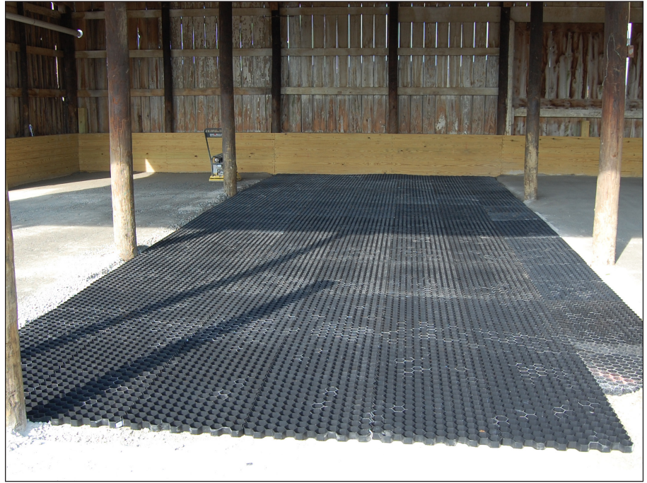
Figure 7. Gravel paver grid used to reinforce a barn floor where livestock will be confined.
