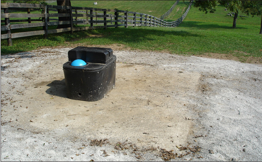
Figure 9. A soil-cement pad placed adjacent to a concrete pad for a waterer.
