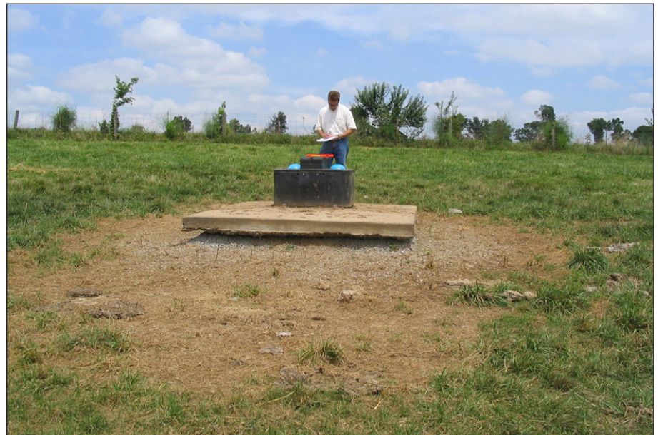
Figure 3. Poorly constructed foundation for a concrete pad that could create too much air flow, which could freeze water pipes.
