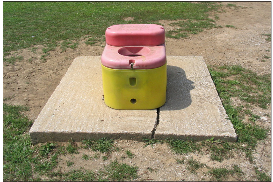
Figure 2. Poorly constructed foundation for a concrete pad.
